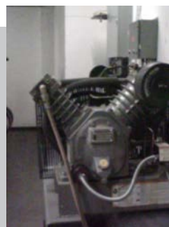
Air Compressor – Full Visible
